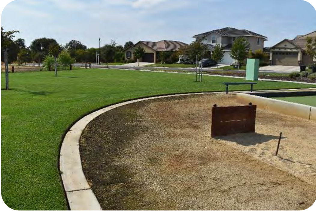
Signs of ponding at RG Phillips Park.
